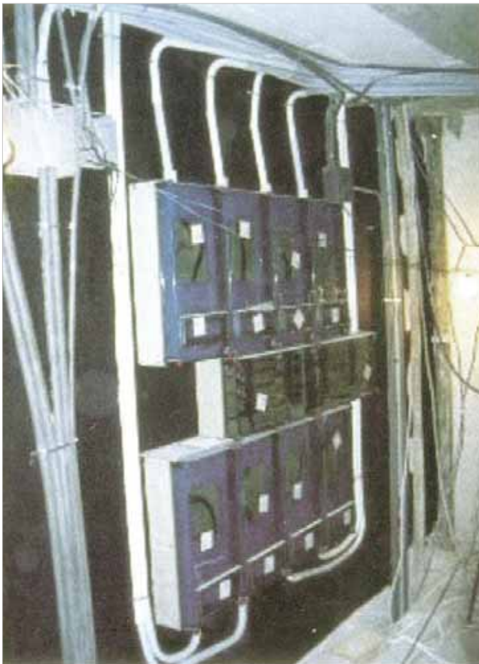
3) Shielding of a power distribution room, adjacent to a childrens bedroom.
